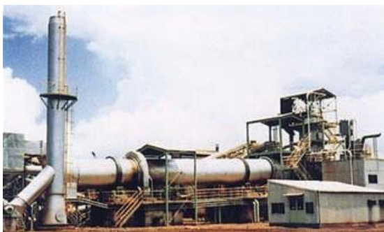
A rotary dryer for the removal of free water
