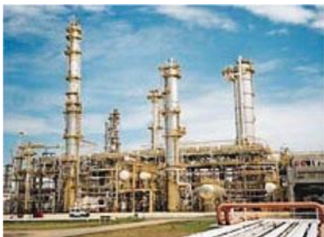
Fluid heating in a petroleum process heater
